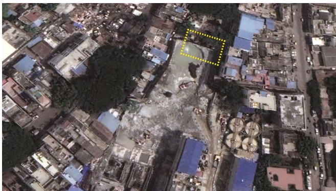
Construction status of Cantonment Metro Station as of end July 2021. BMRCL took possession of land incl. TTCD area on 30 August 2019
